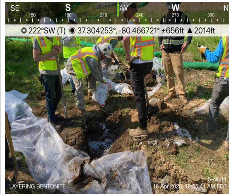
Photo Description: Void was excavated and layered with bentonite and native soil to repair.
