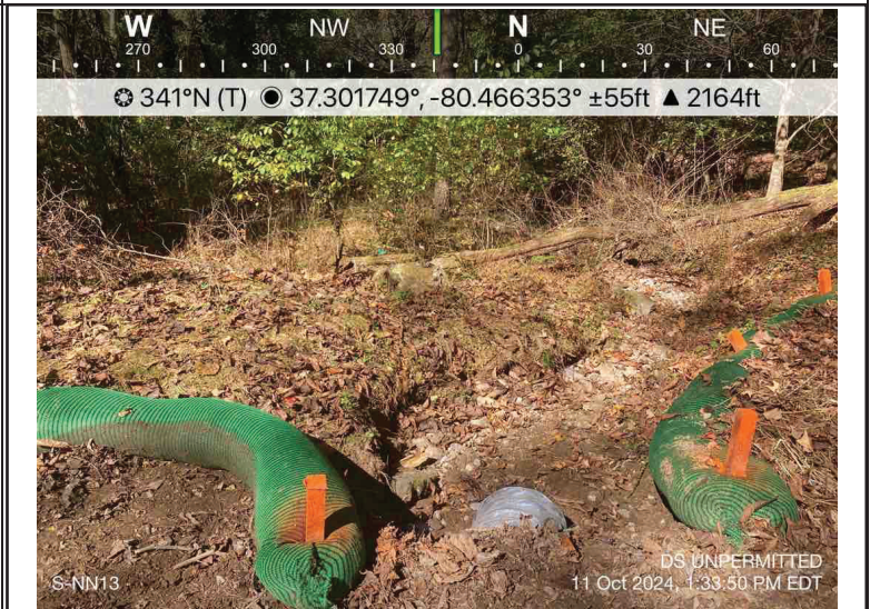
Photo Description: Downstream view of unpermitted area during post-construction assessment.
