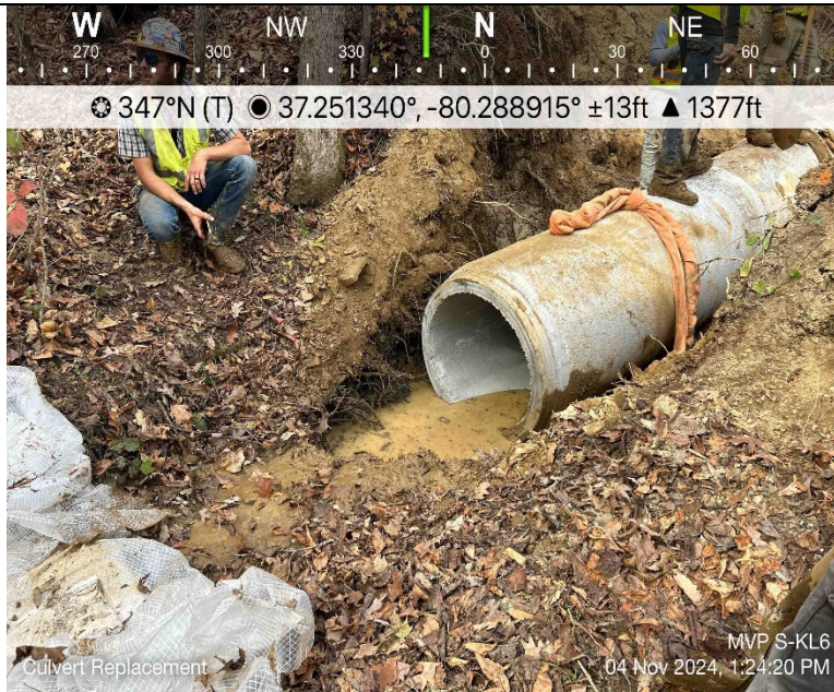
Photo Description: New culvert installed with proper countersinking depth of 6" below natural stream bottom.
