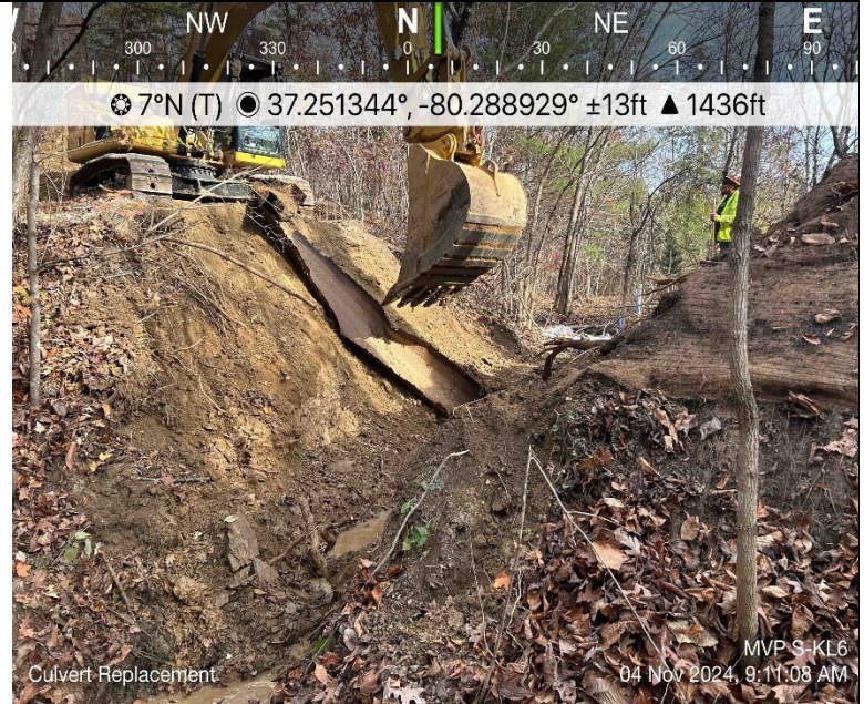
Photo Description: Existing culvert removal. Steel culvert was heavily rusted and disintegrated during removal.
