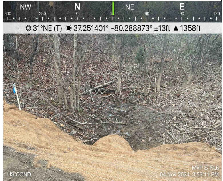
Photo Description: View of upstream conditions from the new culvert installation after final stabilization.
