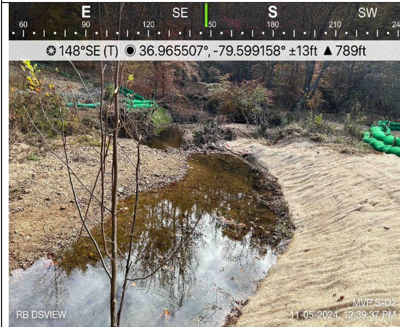
Photo Description: Looking downstream at the right bank. Erosion control matting installed properly.
