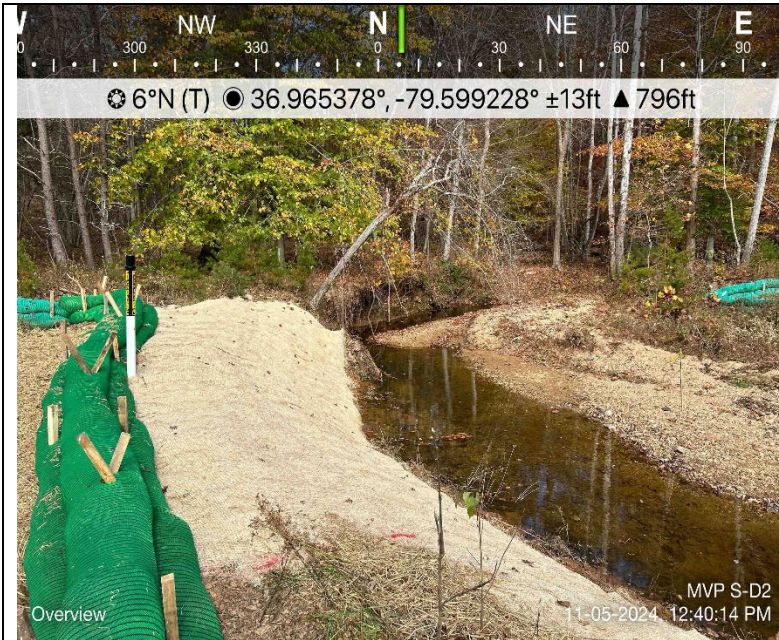
Photo Description: View of regraded bank. Erosion control matting installed, keyed-in, and stapled.
