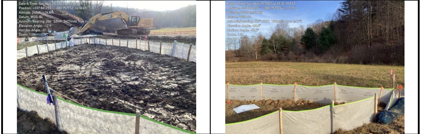
GPS Location See Photo GPS Location See Photo Description View of permitted resource impact area during post-construction assessment. Description At edge of LOD, view of unimpacted resource area conditions during post-construction assessment.
