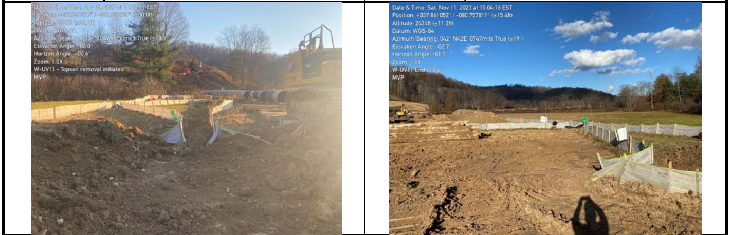
GPS Location See Photo GPS Location See Photo Description Photo 1: Removal of first 12 inches of topsoil in the northwestern corner of the aquatic resource. Description Photo 2: Remainder of the first 12 inches of topsoil in the aquatic resource removed.
