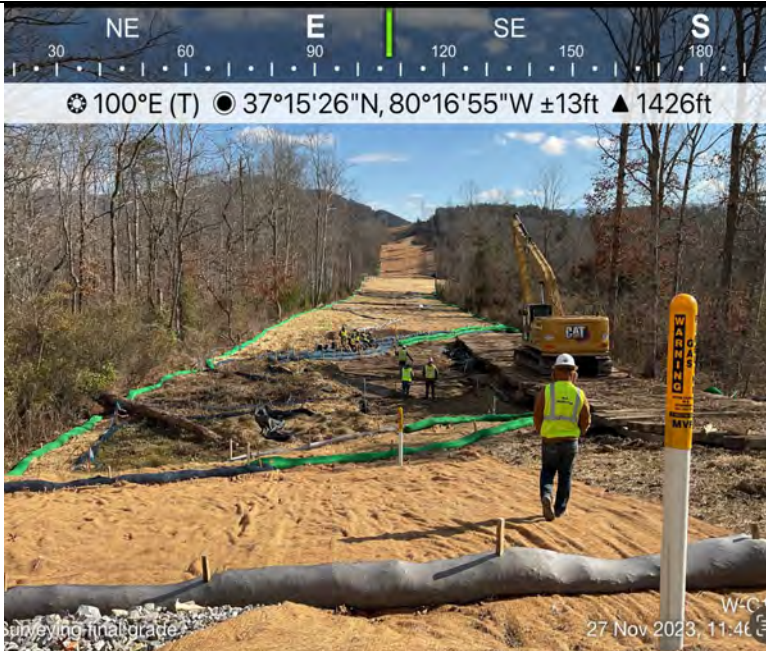
Photo Description: Survey conducting as-built shots to confirm that the wetland meets pre-construction conditions.
