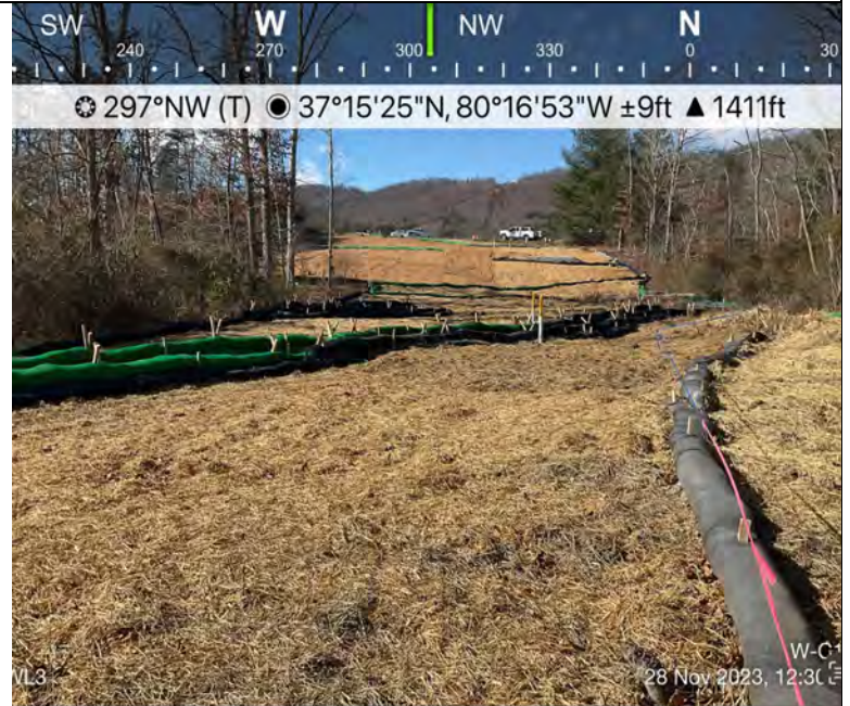
Photo Description: Final conditions and an overview of the wetland after construction was complete.
