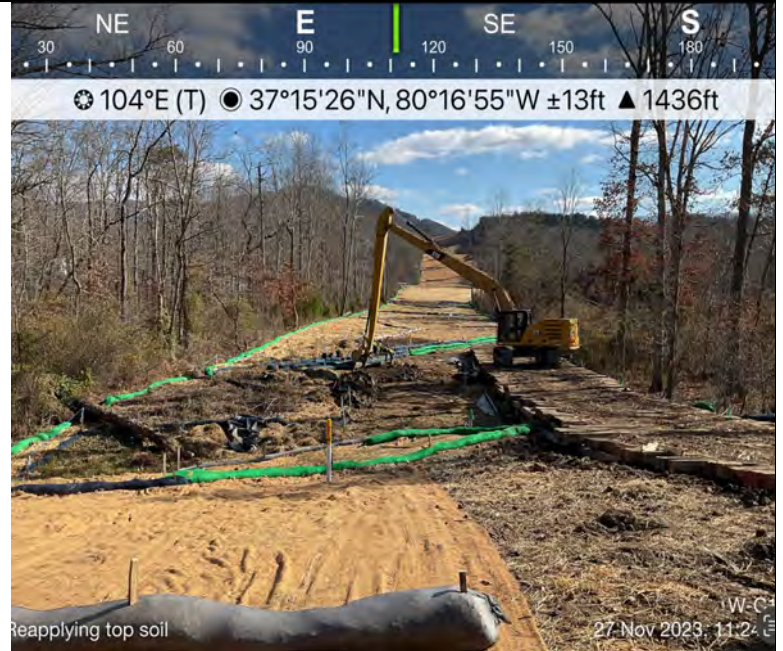
Photo Description: Topsoil being replaced after fill material was used to fix the impacted section of the wetland.
