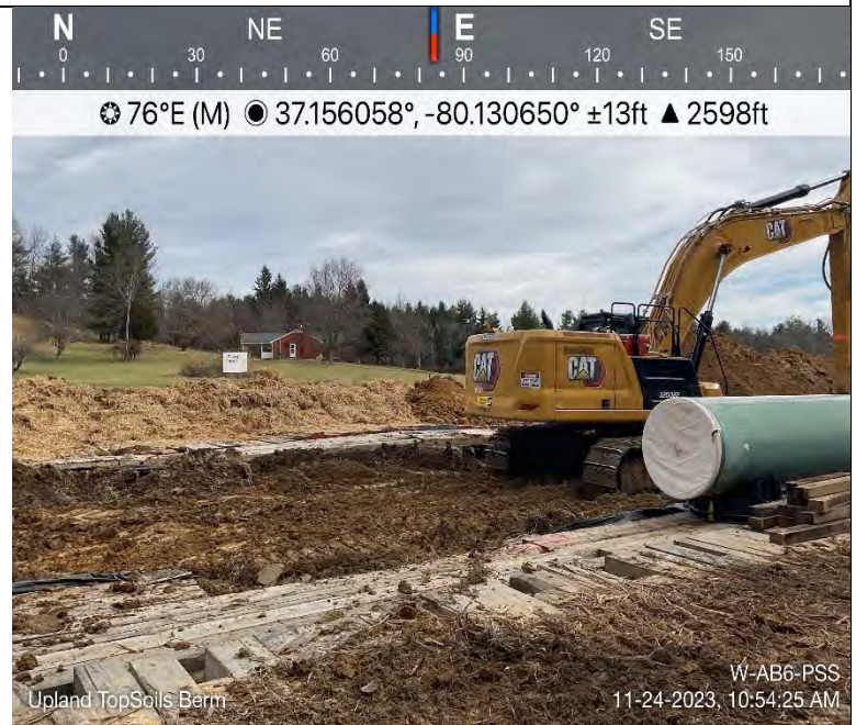
Photo Description: Topsoil and subsoil berms across from trenching area. Stockpiles stabilized.
