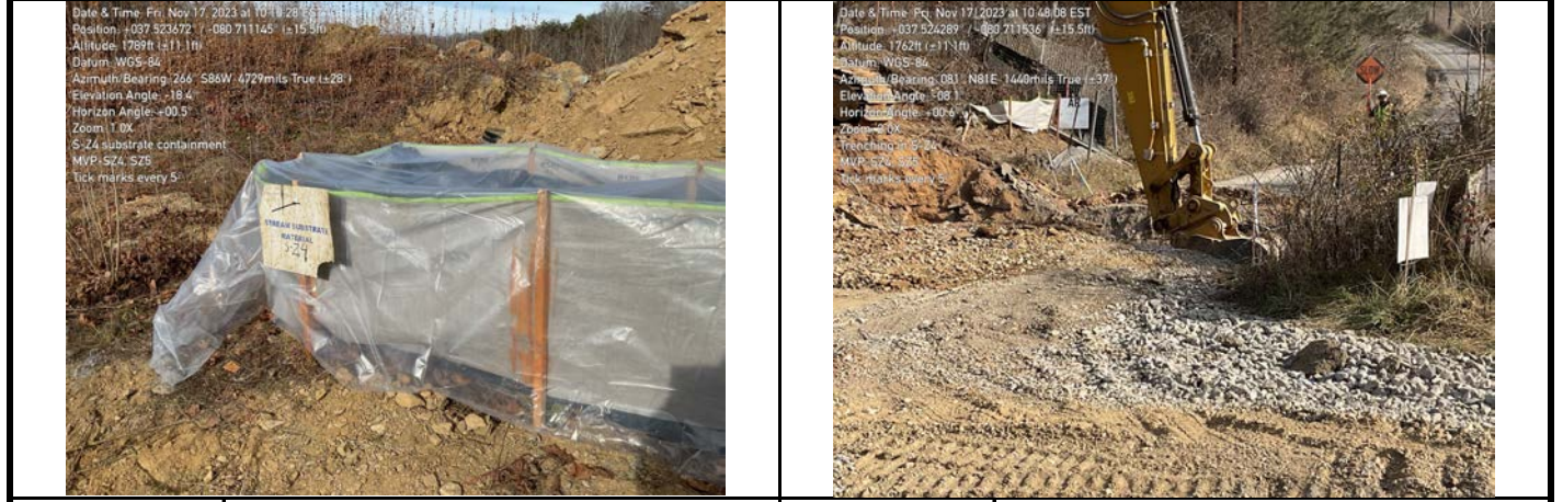
GPS Location See Photo GPS Location See Photo Description Photo 1: Stream substrate containment structure. Description Photo 2: Trenching through resource.
