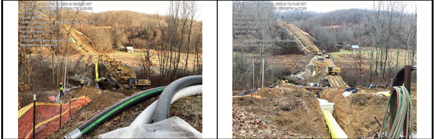
GPS Location See Photo GPS Location See Photo Description Photo 5: Lowering pipe into trench through aquatic resource area. Description Photo 6: Backfilling and trench breaker construction.
