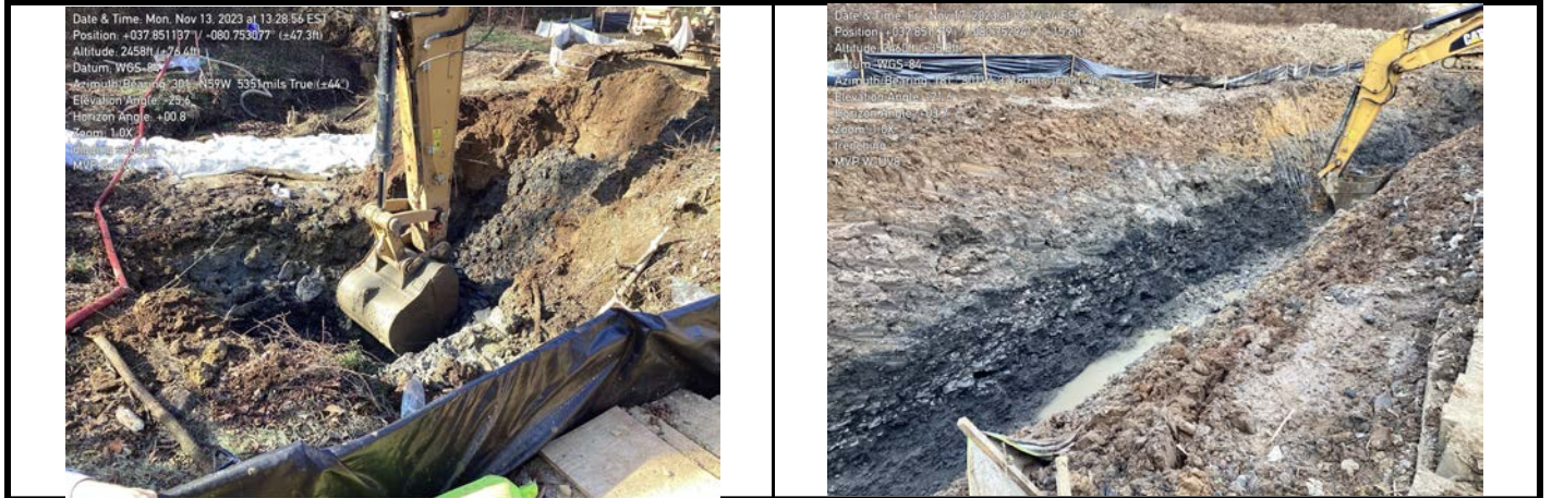
GPS Location See Photo GPS Location See Photo Description Photo 3: Excavating trench in aquatic resource area. Description Photo 4: Excavating trench.
