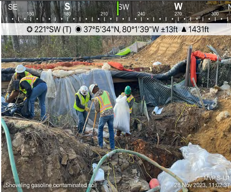
Photo Description: The crew removing the contaminated soil after the equipment malfunctioned.
