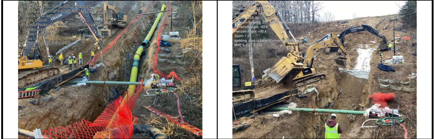
GPS Location See Photo GPS Location See Photo Description Photo 5: Pipe lowered into trench and flume pipe restored. Description Photo 6: Padding and backfilling of trench. Completed trench breaker.
