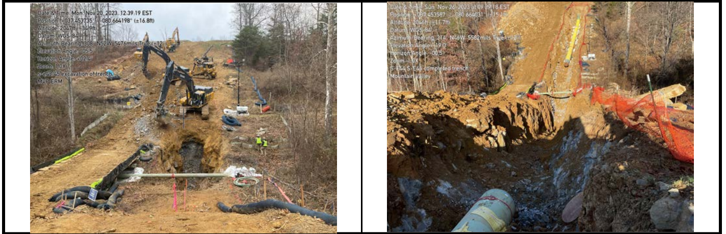
GPS Location See Photo GPS Location See Photo Description Photo 3: Excavating trench. Description Photo 4: Excavation of trench through aquatic resources and buffer complete.
