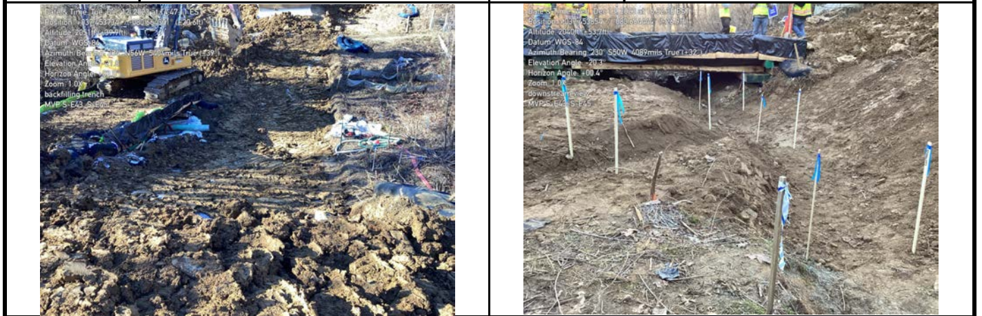
GPS Location See Photo GPS Location See Photo Description Photo 7: Backfilling trench. Description Photo 8: OHWM staked by survey crew.
