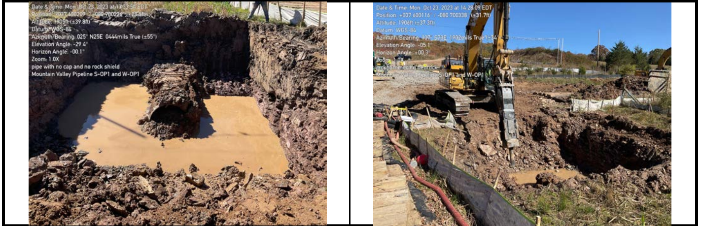
GPS Location See Photo GPS Location See Photo Description Photo 3: Exposed pipe in aquatic resource. Description Photo 4: Hammering in aquatic resource.
