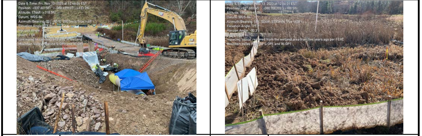
GPS Location See Photo GPS Location See Photo Description Photo 7: Backfilling and constructing trench breaker outside of aquatic resource. Description Photo 8: Restoring wetland topsoil removed during 2018 construction as per FERC instruction.
