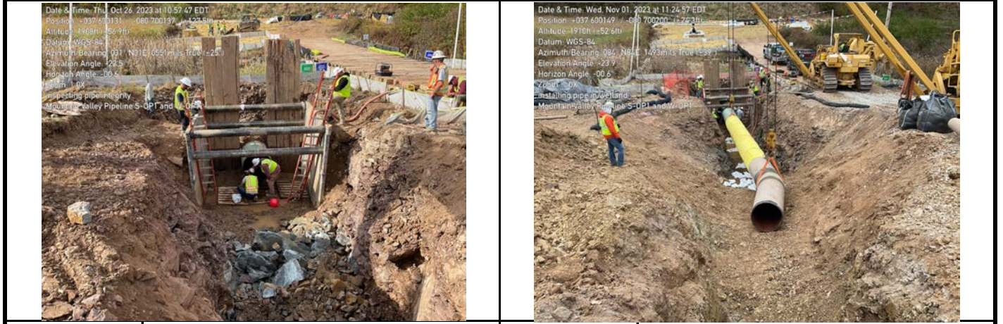
GPS Location See Photo GPS Location See Photo Description Photo 5: Pipe inspection. Description Photo 6: Installing pipe in trench in aquatic resource area.
