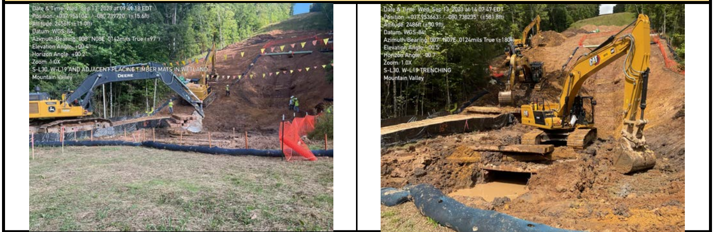
GPS Location See Photo GPS Location See Photo Description Photo 3: Adjusting timber mats for work in wetland. Description Photo 4: Trenching in aquatic resource from timber mats.
