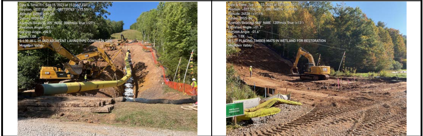
GPS Location See Photo GPS Location See Photo Description Photo 5: Installation of south trench breaker between S-L22 and W-L19. Description Photo 6: Restoration of wetland 12" topsoil to resource.
