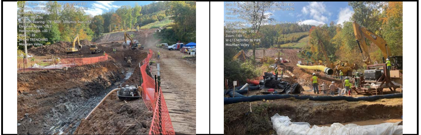
GPS Location See Photo GPS Location See Photo Description Photo 3: Trench completed through aquatic resource and upland pipe exposed. Description Photo 4: Lowering pipe into trench in aquatic resource area.
