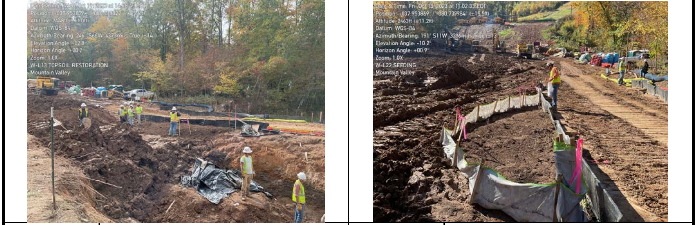
GPS Location See Photo GPS Location See Photo Description Photo 7: Survey verifying final grade and location of restored (topsoiled) wetland resource. Description Photo 8: Seeding of wetland resource.
