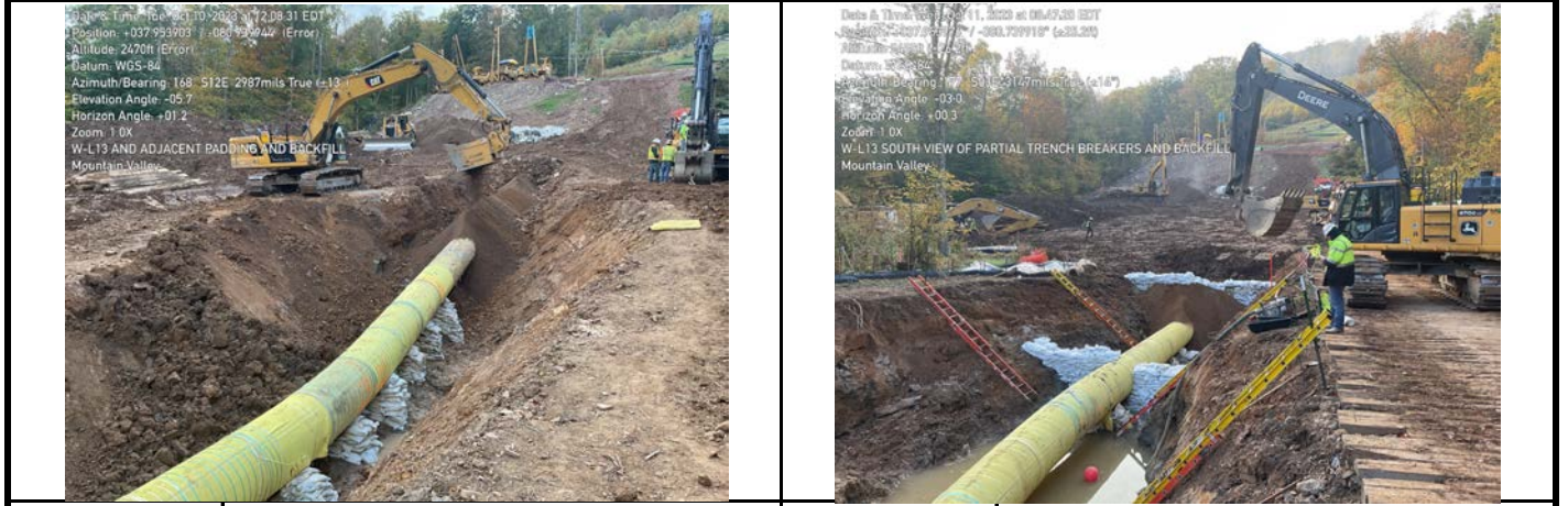
GPS Location See Photo GPS Location See Photo Description Photo 5: Sifting and backfilling of trench in aquatic resource area. Description Photo 6: Construction of trench breakers adjacent to aquatic resource area.
