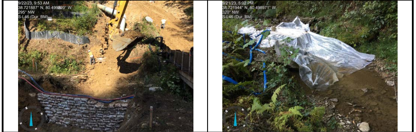
GPS Location See photo GPS Location See photo Description Padding the pipe after trench breaker installation. Description Dam and pump outflow downstream off ROW. Clear water, no scouring or erosion.
