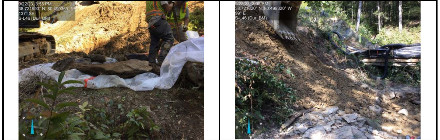
GPS Location See photo GPS Location See photo Description GPS boulders stored in plastic are now being placed back in the stream. Description Rebuilding the stream banks.
