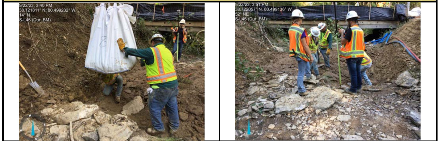
GPS Location See photo GPS Location See photo Description Replacing stream bed substrate, in the reverse order they were removed. Description Replacing stream bed substrate, and GPS located prominent boulders.
