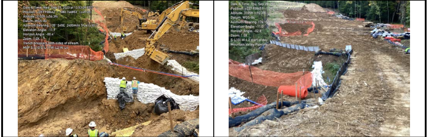
GPS Location See Photo GPS Location See Photo Description Photo 5: Filling of trench and construction of trench breakers. Description Photo 6: Filling of trench in aquatic resource area complete.
