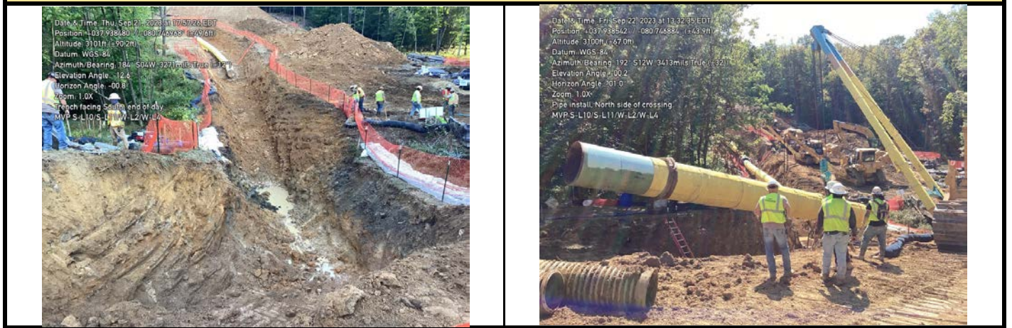
GPS Location See Photo GPS Location See Photo Description Photo 3: Trenching through aquatic resources. Description Photo 4: Pipe being placed in trench.
