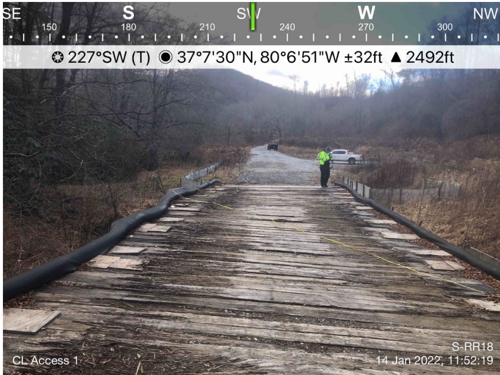
Photo Type: CL ACCESS 1 Location, Orientation, Photographer Initials: Standing in Access Road looking SW, KB
