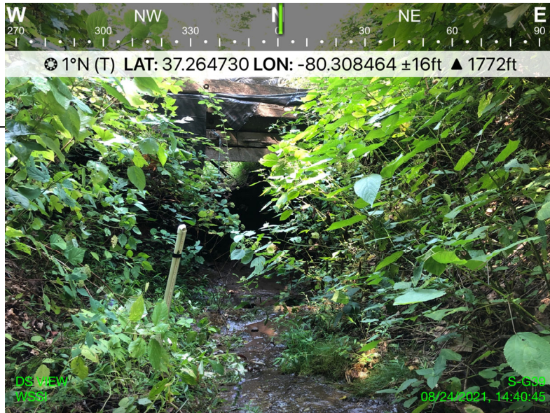
Standing upstream looking N downstream within the ROW. Assessment is limited to areas within the temporary ROW.
