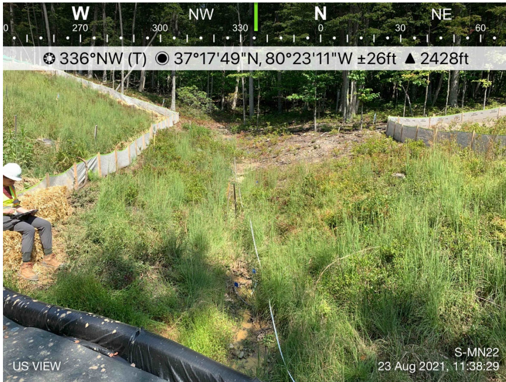
Photo Type: US VIEW Location, Orientation, Photographer Initials: Upstream view of ROW looking N, TC
