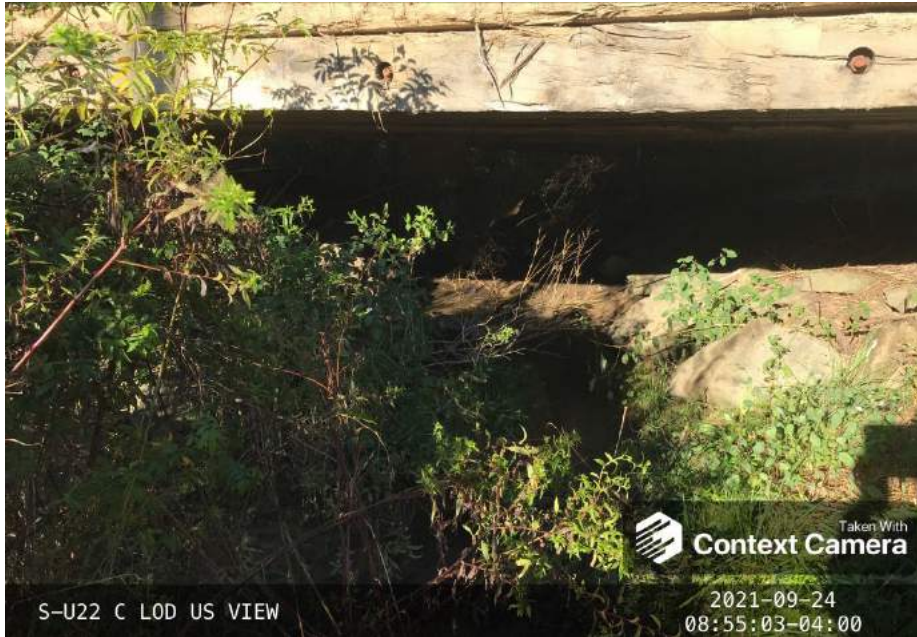
Photo Type: US View at Center Location, Orientation, Photographer Initials: Center ROW, Upstream View, RH/VM Lat: 37.839558 Long: -80.748496
