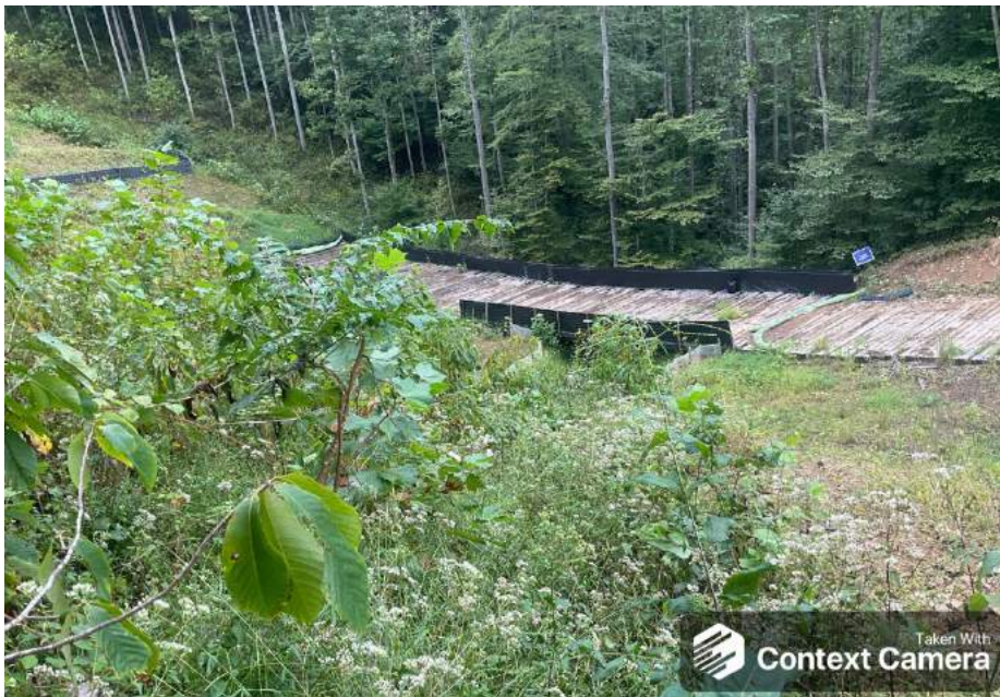
Photo Type: US, DS View Location, Orientation, Photographer Initials: Upstream Edge of ROW, Downstream View, KY/ZS Lat: 38.67211, Long: -80.476515
