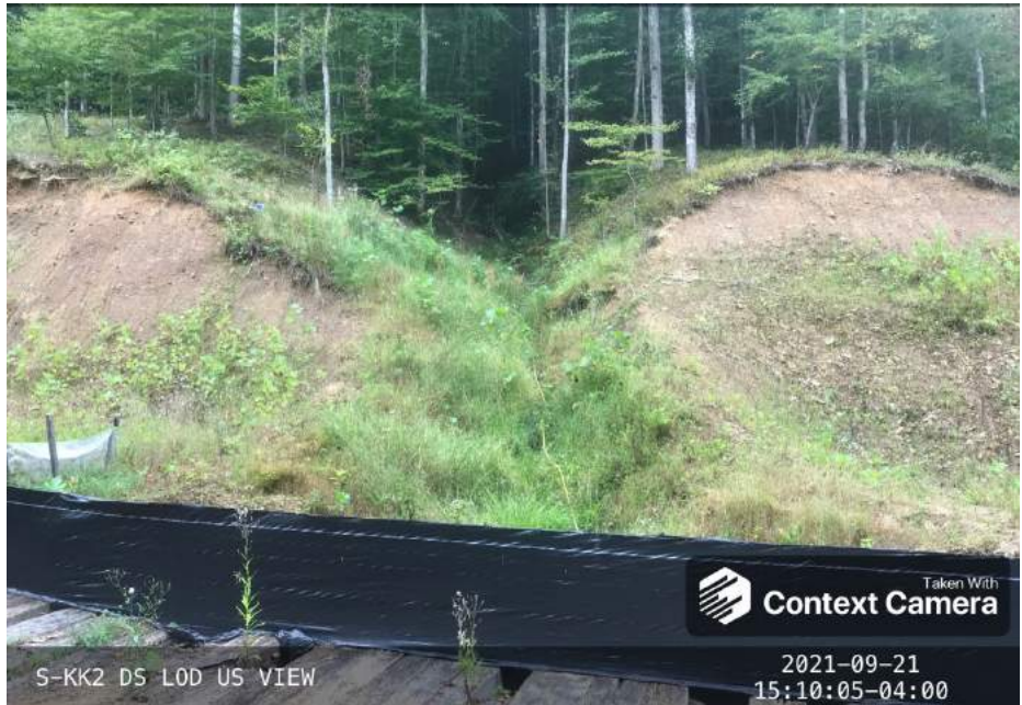
Photo Type: DS, US View Location, Orientation, Photographer Initials: Downstream Edge of ROW, Upstream View, RH/VM Lat: 38.672226 Long: -80.476315
