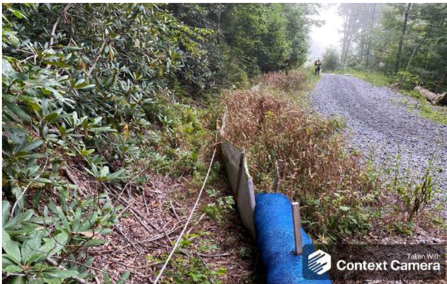
Photo Type: US, DS View Location, Orientation, Photographer Initials: Upstream Edge of ROW, Downstream View, COC Lat: 38.309738 Long: -80.675733
