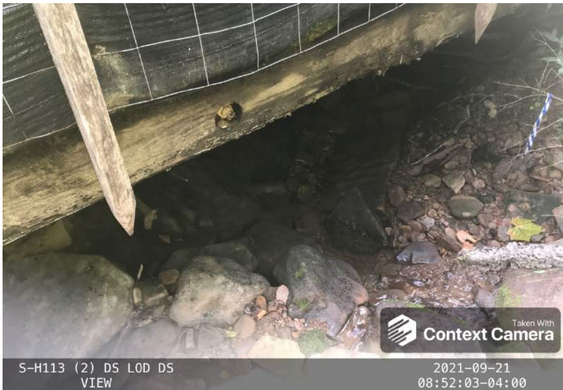
Photo Type: DS, DS View Location, Orientation, Photographer Initials: Downstream Edge of ROW, Downstream View, RH, VM Lat: 38.612878 Long: -80.503687
