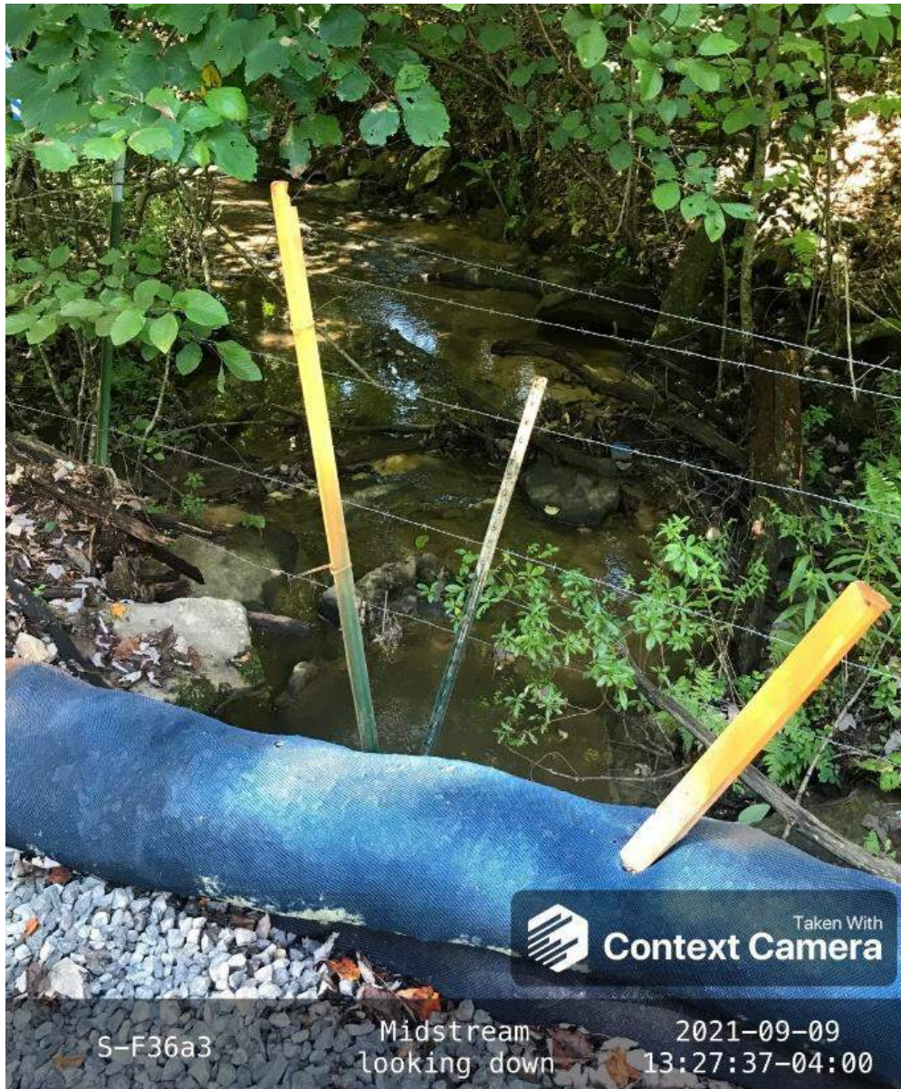
Photo Type: DS View at Center Location, Orientation, Photographer Initials: ROW Center, Downstream View, EG Lat: 38.418662 Long: -80.573898
