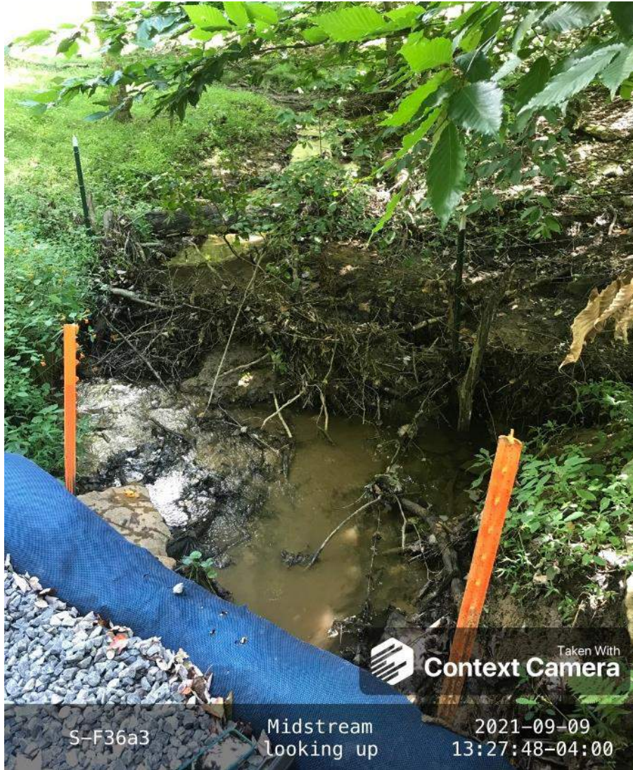
Photo Type: US View at Center Location, Orientation, Photographer Initials: Center ROW, Upstream View, EG Lat: 38.418662 Long: -80.573898
