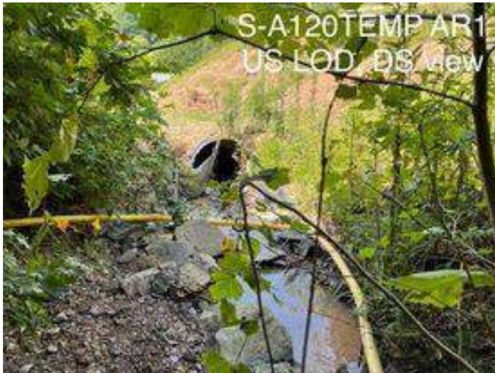
Photo Type: US, DS View Location, Orientation, Photographer Initials: Upstream Edge of ROW, Downstream View, BC/DP Lat:39.489914 Long: -80.522135
