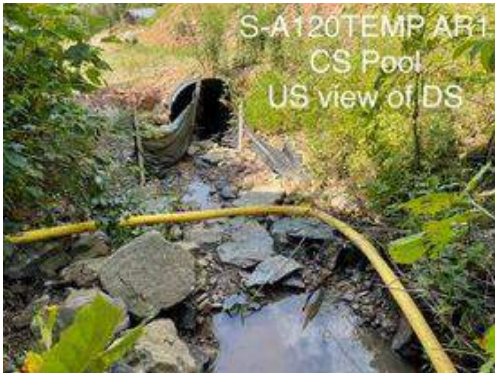
Photo Type: Pool, US View Location, Orientation, Photographer Initials: Downstream of Pool, Upstream View, BC/DP Lat:39.489914 Long: -80.522135
