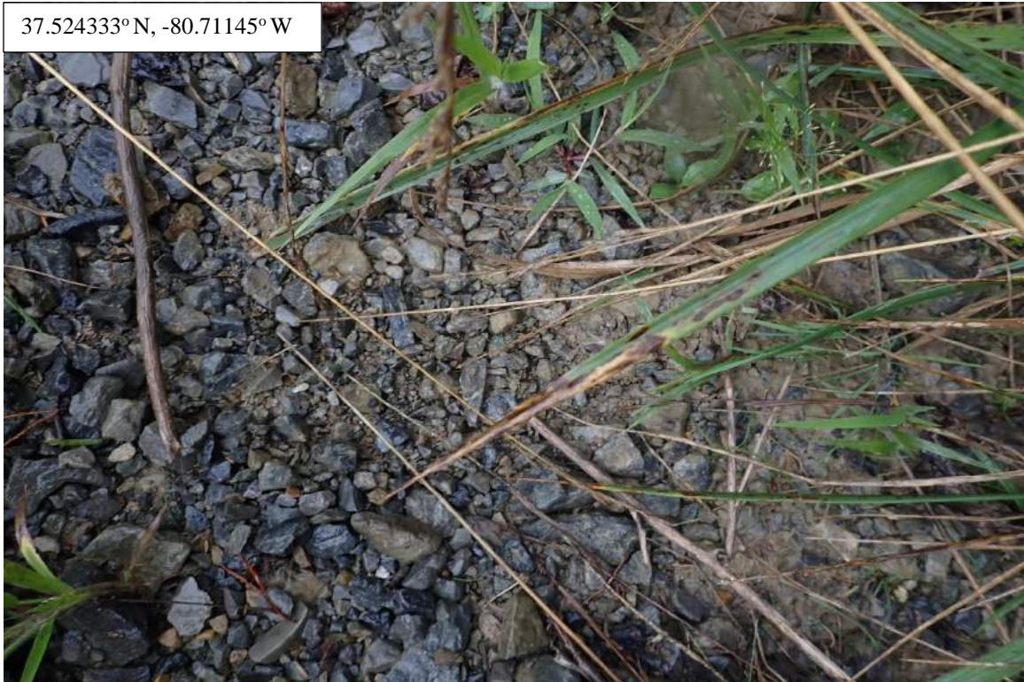
Photo Type: View of Substrate Location, Orientation, Photographer Initials: View of Substrate, AK/TA/SM
