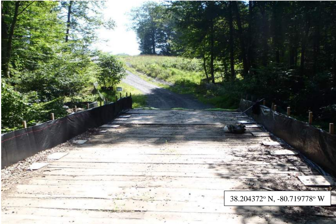
Photo Type: Facing W Across Bridge Location, Orientation, Photographer Initials: Facing West Across Bridge, TF/AG/WP/EW
