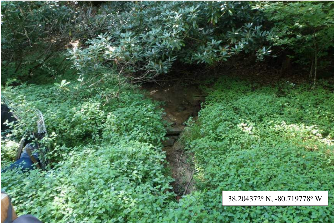
Photo Type: US View at US Side of Bridge Location, Orientation, Photographer Initials: Upstream Side of Bridge, Upstream View, TF/AG/WP/EW
