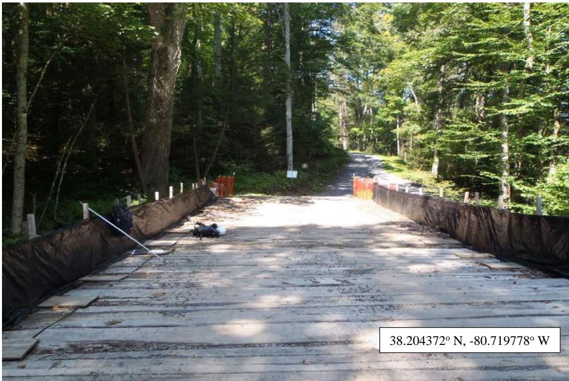
Photo Type: Facing N Across Bridge Location, Orientation, Photographer Initials: Facing North Across Bridge, TF/AG/WP/EW
