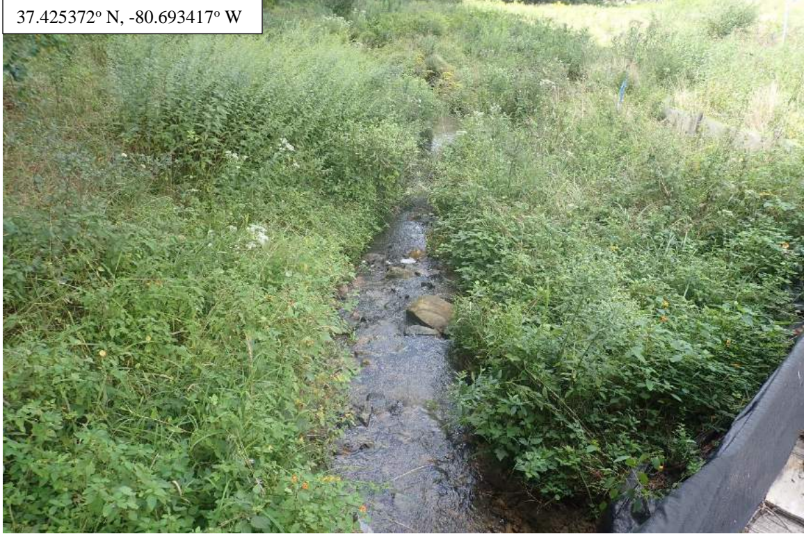
Photo Type: DS Edge of TMB, DS View Location, Orientation, Photographer Initials: Downstream Edge of Bridge, Downstream View, AK/TF (8/18/2021)
